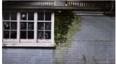
Penetrating damp becomes more noticeable when it rains
