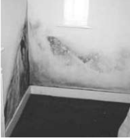
Walls with black mould growth
