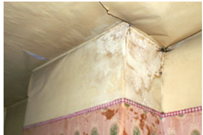
Internal penetrating damp
