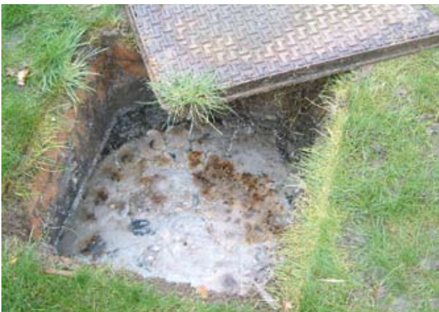
Fat building up in a manhole.
