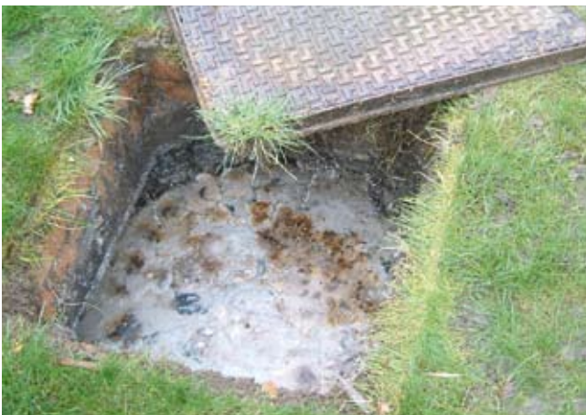
Fat building up in a manhole.
