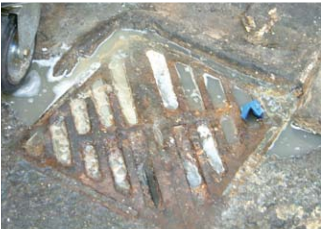
A drain gully blocked with fat.
