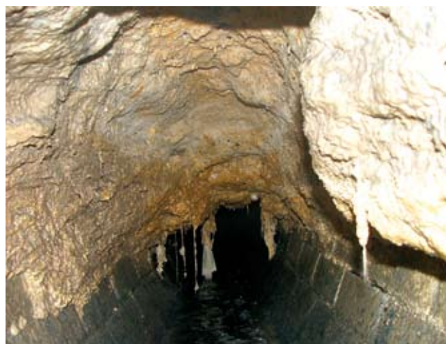
Build up of fat in sewer.
