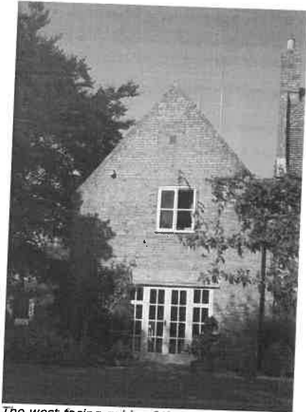
The west facing gable of the north pavilion. Note the blocked window beneath the apex of the gable, the reduced window below and replacement French windows and brickwork of the removed wooden lintel.
