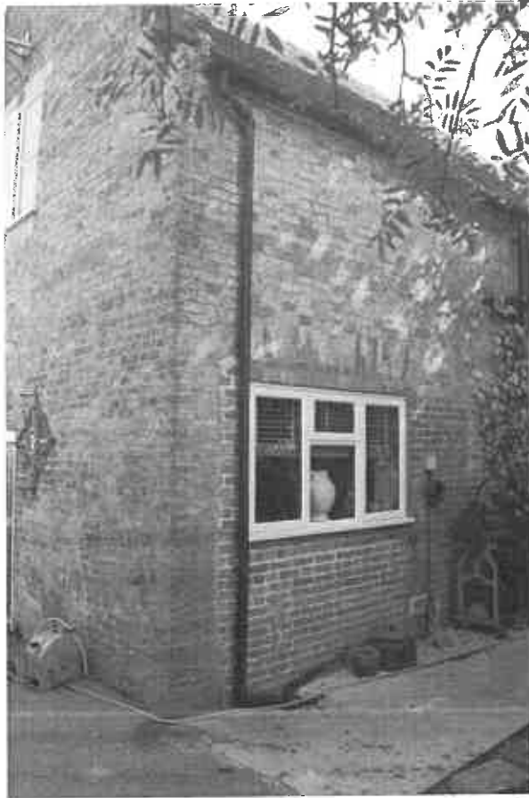
The rear elevation of the northern pavilion showing the blocked and glazed, possibly former carriage entrance.
