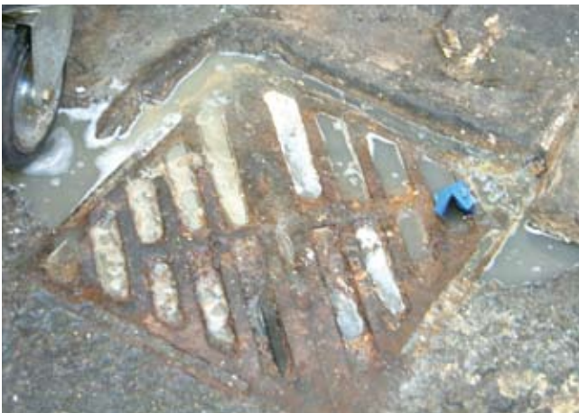
A drain gully blocked with fat.
