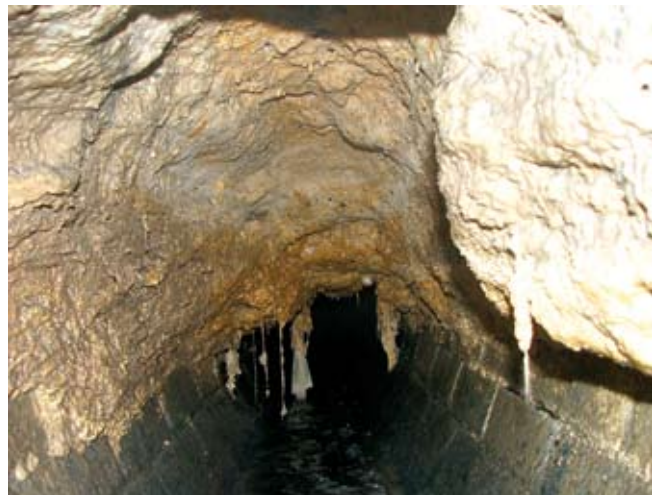
Build up of fat in sewer.
