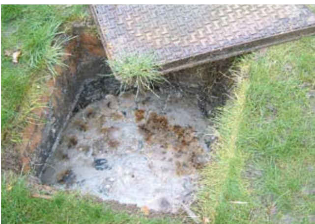
Fat building up in a manhole.
